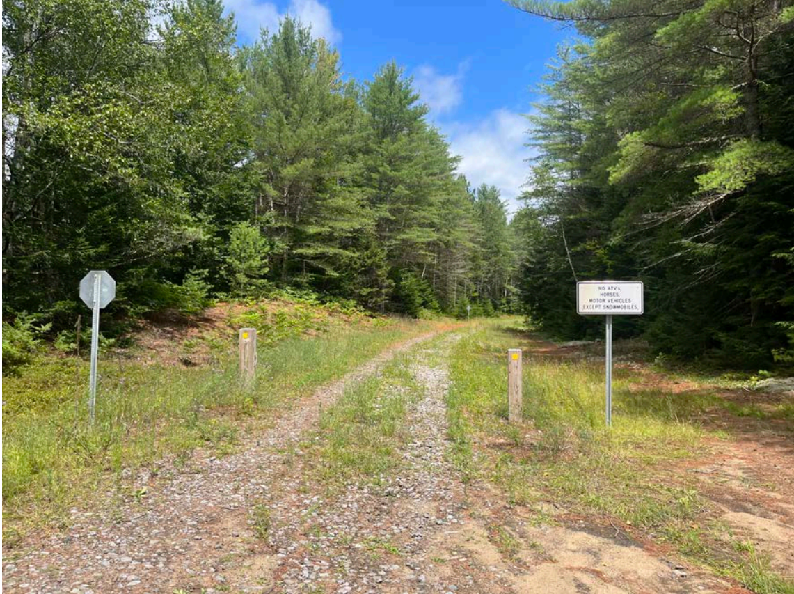
This photograph was taken on Phase 3 of the Adirondack Rail Trail to the west of Rollins Pond at the intersection with Floodwood Reservation Road. It shows that the existing railbed is approximately 10 feet wide or more and there is plenty of cleared space on both sides of the railbed. The bollards and signage are already in place.
