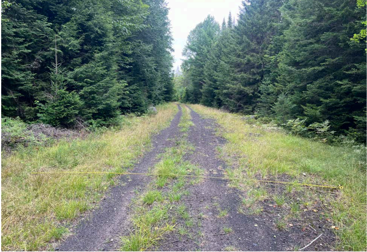
This photograph was taken on Phase 3 of the Adirondack Rail Trail to the west of Rollins Pond. It shows that the existing railbed is approximately 10 feet wide or more and there is plenty of cleared space on both sides of the railbed. The total width of the cleared area was more than 20'.
